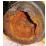
▲ Figure 16.5 A biofilm fouling the insides of a pipe
